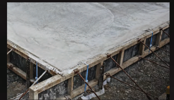
2 RibRaft RaftMix® concrete is poured level with the form work leaving the top of the HotEdge Extra® panel uncovered. The HotEdge® panels for brick cladding should be positioned 25mm below the rebate former to create a ledge covering the beveled top of the panel to support brick veneers.
