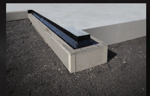
3 Boxing is removed, revealing a truly integrated, aesthetically finished thermal barrier to help achieve H1 compliance. Firth recommend two coats of acrylic paint should be applied to all exposed surfaces for optimum service life and insulation. NOTE: Images shows both HotEdge® (with rebate for brick veneers) and HotEdge Extra® (for non-brick cladding).
